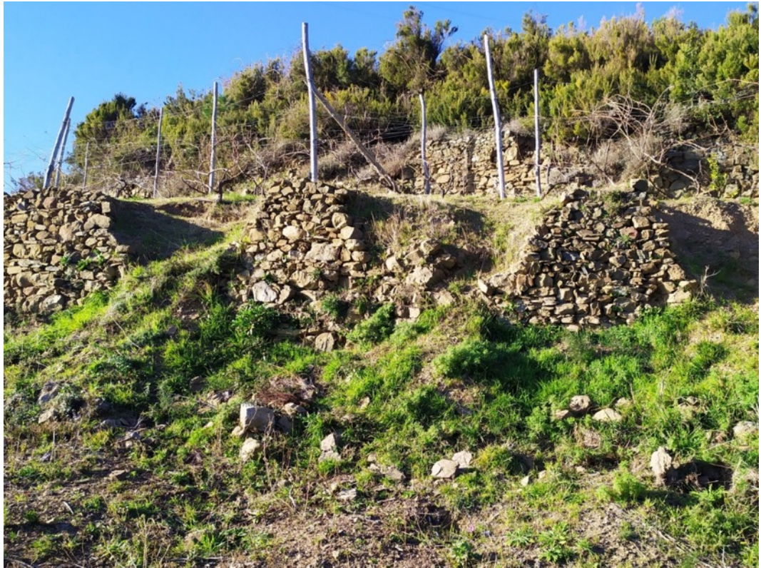
Figure 12 Partial collapse (upper portion of the dry-stone wall)
