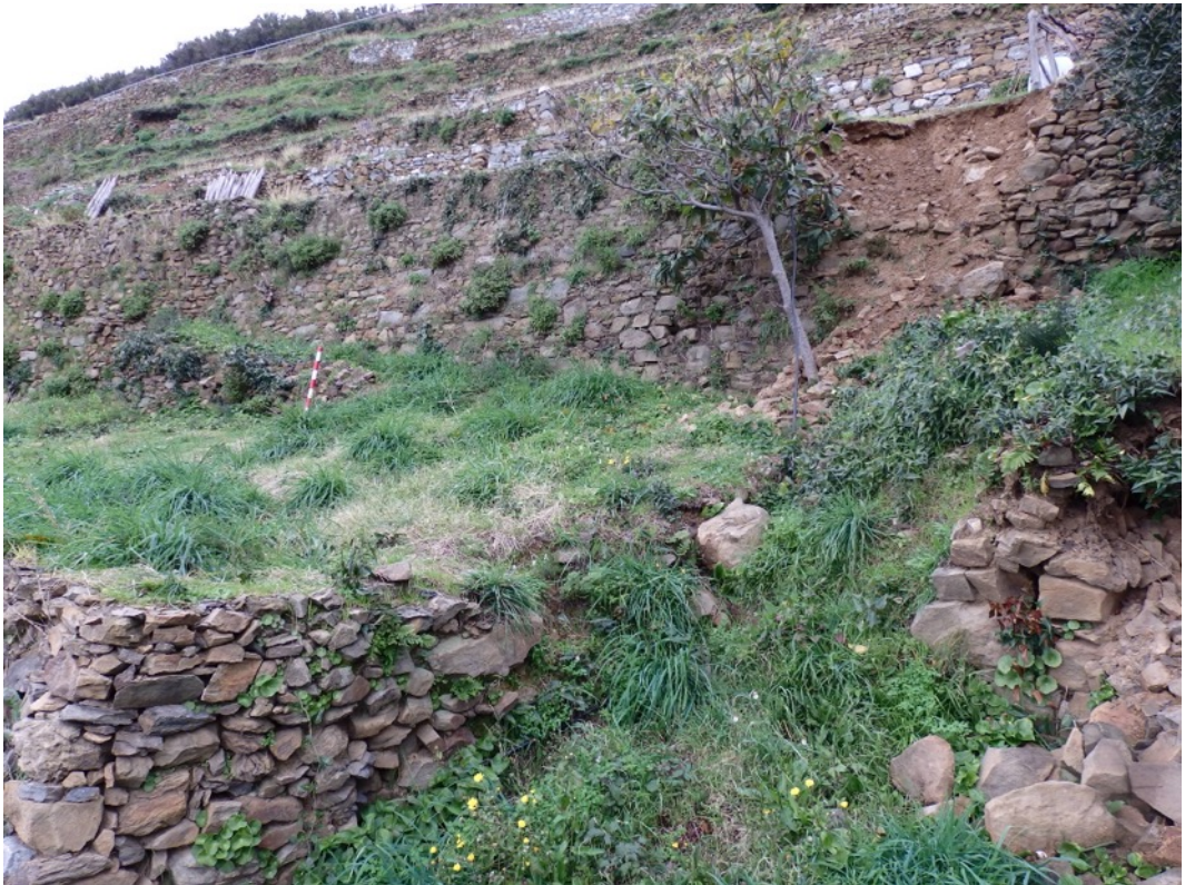
Figure 15 An un-maintained drain channel
